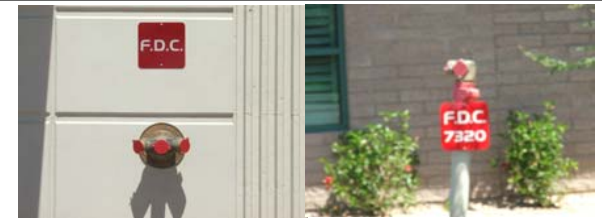
Fire Department Connections clearly marked
