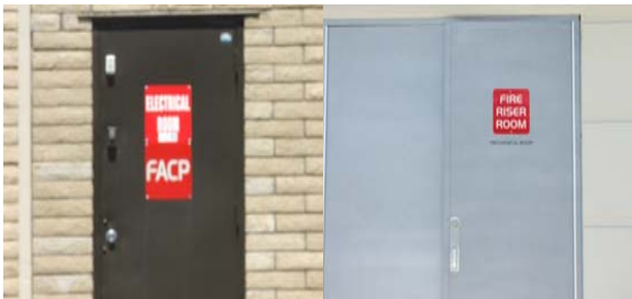
Fire Alarm and Riser Room doors should be labeled.
