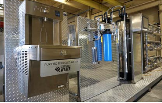
Purified Drinking Water demonstration station
