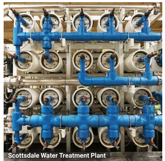
Scottsdale employee inspects the technological infrastructure at Scottsdale Water
