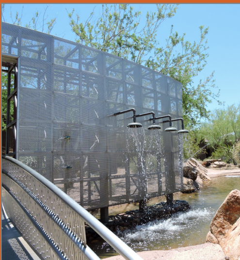
The CAP Water Treatment Plants are located at the Scottsdale Water Campus in north Scottsdale.
